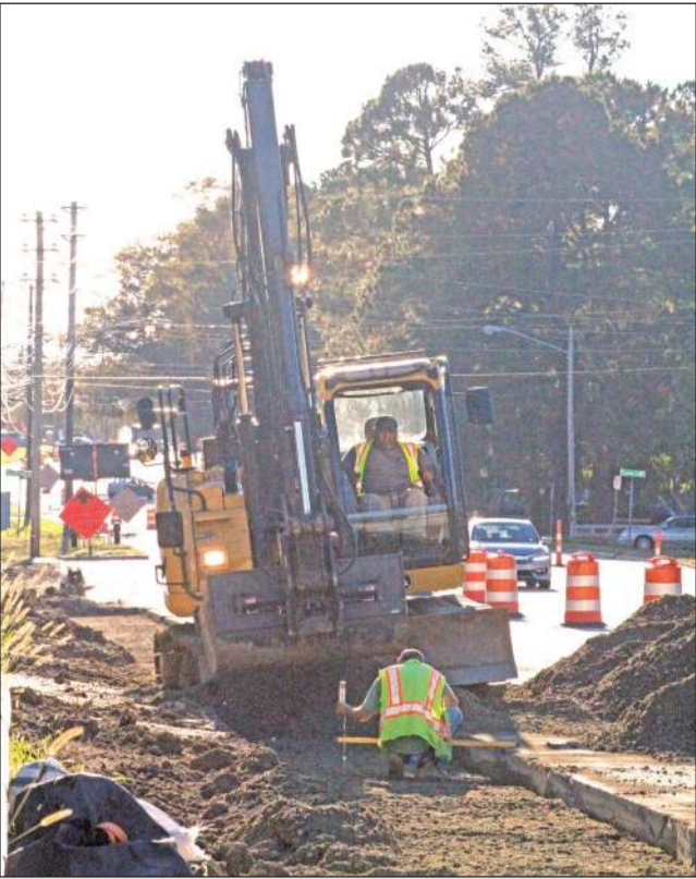
S.T. Wooten Corp. operators Juan Carlos Limon and Patrick Callon work Wednesday on digging a ditch along Herring Avenue to add sidewalks as part of the infrastructure improvement project nearby on U.S. 301. Brie Handgraaf | Times
